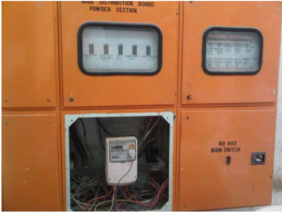
Figure 4.17: Distribution Board for Powder section and submeter
