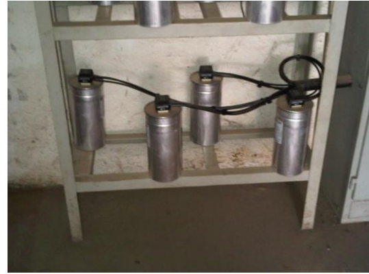
Figure 4.9: Set of Capacitor Banks installed
