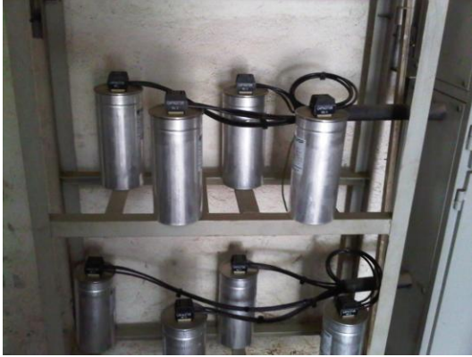
Figure 4.8: New capacitor banks for pf correction.
