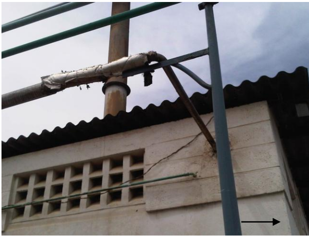
Figure 4.28: Poor or no lagging of steam distribution pipes.
