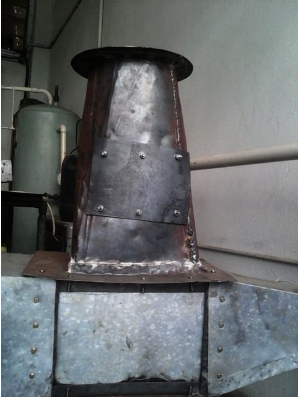
Gas side outlet duct
