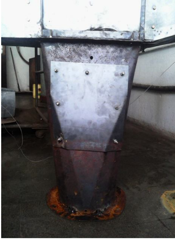
Gas side inlet duct.
